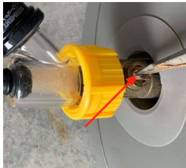
Valve is in ON position
