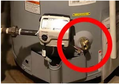
Drain Valve on this gas water heater
