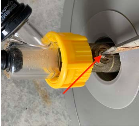
Drain Valve Turned on in line with Sediment Buster™
